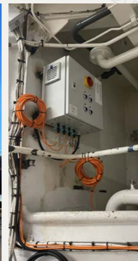
Control unit installed
