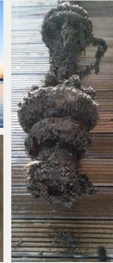
Water intake pipe before Shipsonic fouling protection was installed
