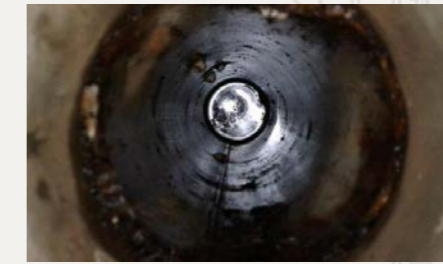
Water intake pipe must be clean before installation
